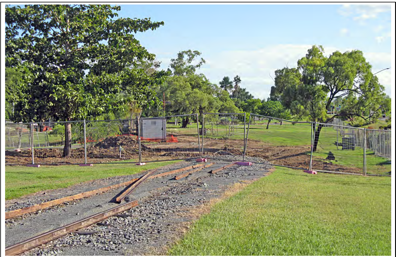
End of rail: Kershaw Gardens' rail line being removed as part of cyclone Marcia restorations, 12 March 2017. The two photos were taken from roughly the same location; the windmill, visible in the photo above, survived the cyclone and is hidden by the trees. The Gardens' relocated (but never restored) North Rockhampton station has also been demolished. Lynn Zelmer photographer [lz_3882-KershawRailway.jpg]
