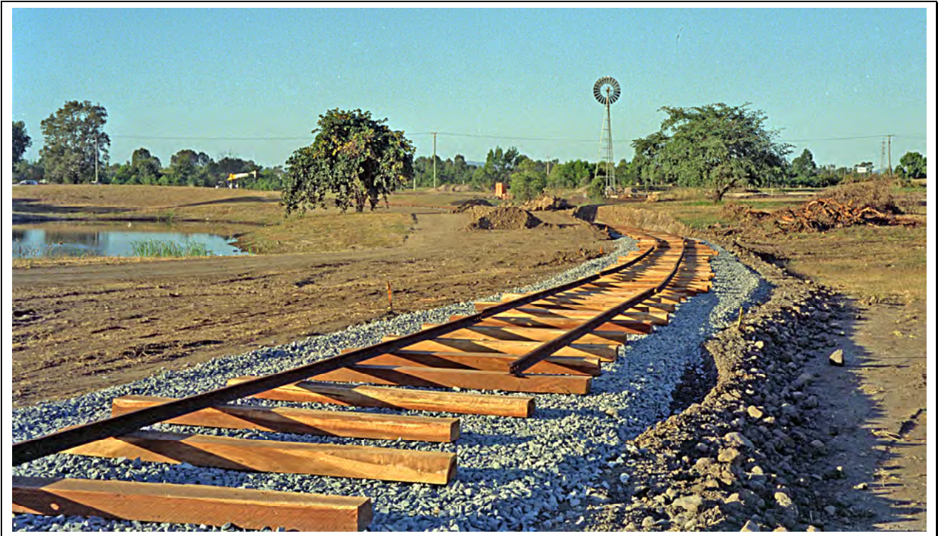
Rails being laid in Kershaw Gardens c1989 when it was proposed that the tram would operate in the park on special occasions. Lynn Zelmer photographer [20FE8108FA5611D8.jpg]
