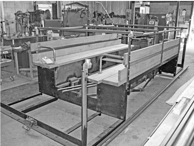
Third carriage for 'Mary Ann' under construction, the metal frame will eventually be raised for the roof structure.
